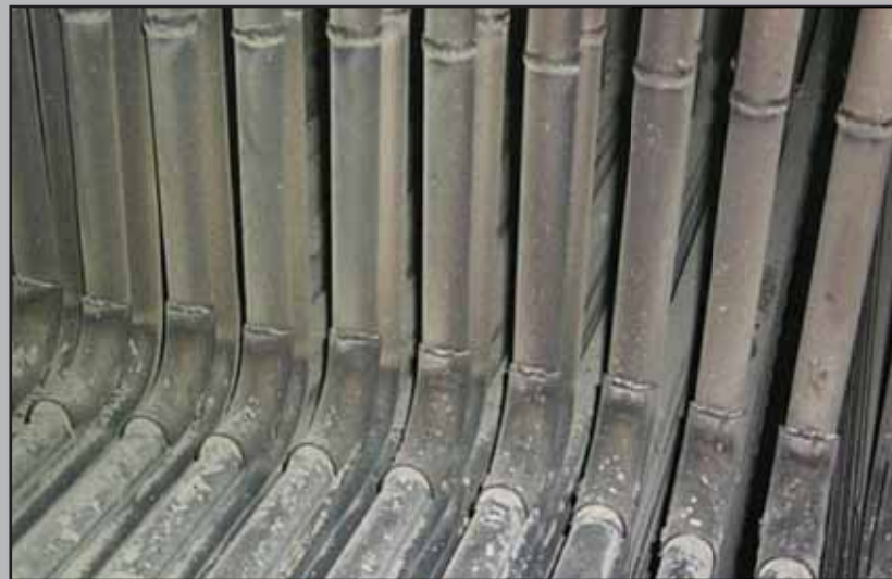
Convection Pass 1300 MW
